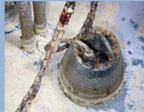
One of two SE pumps for pumping wastewater containing chemicals with large variations in pH from the CIP process at a dairy producing cheese.
